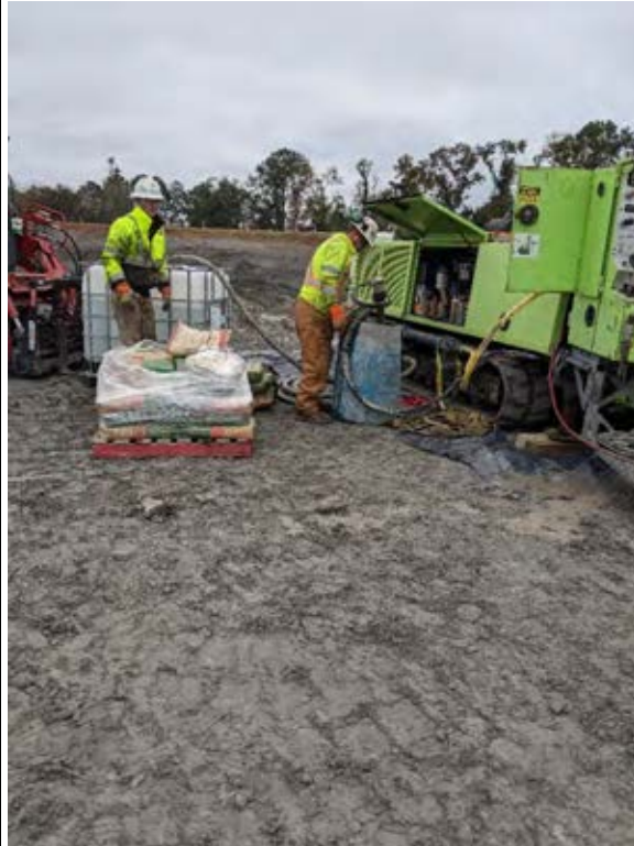
Mixing grout to backfill borehole to bottom of ash pond. Approximately 26.5 gallons
