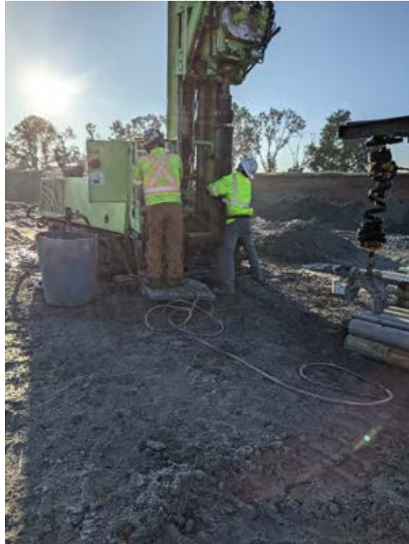
Overdrilling outer casing with 9-inch augers in upper 25 ft of the well down to bottom of ash pond.
