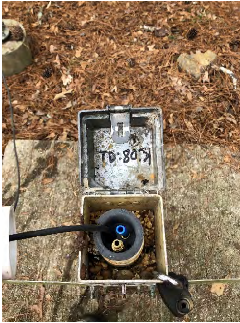
Photo #1: Dedicated pump Installed
