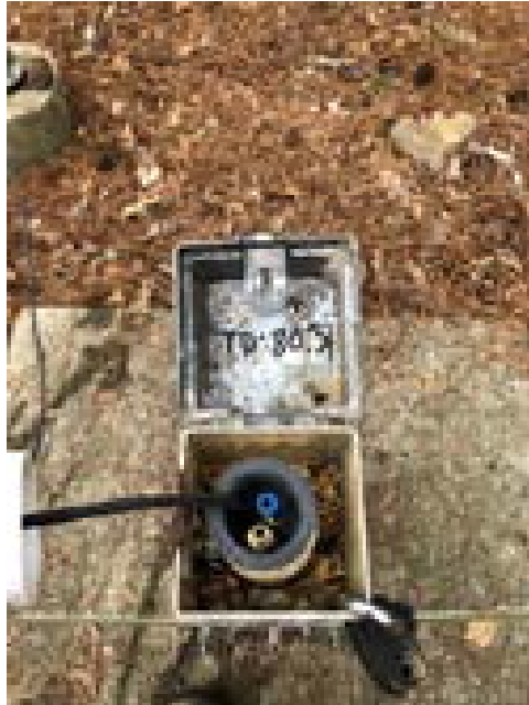
Photo #1: Dedicated pump Installed
