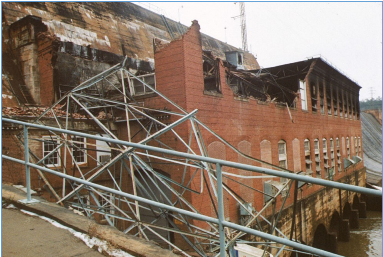
Figure 8. Lloyd Shoals powerhouse damaged in 1983 fire (Courtesy of Georgia Power).
