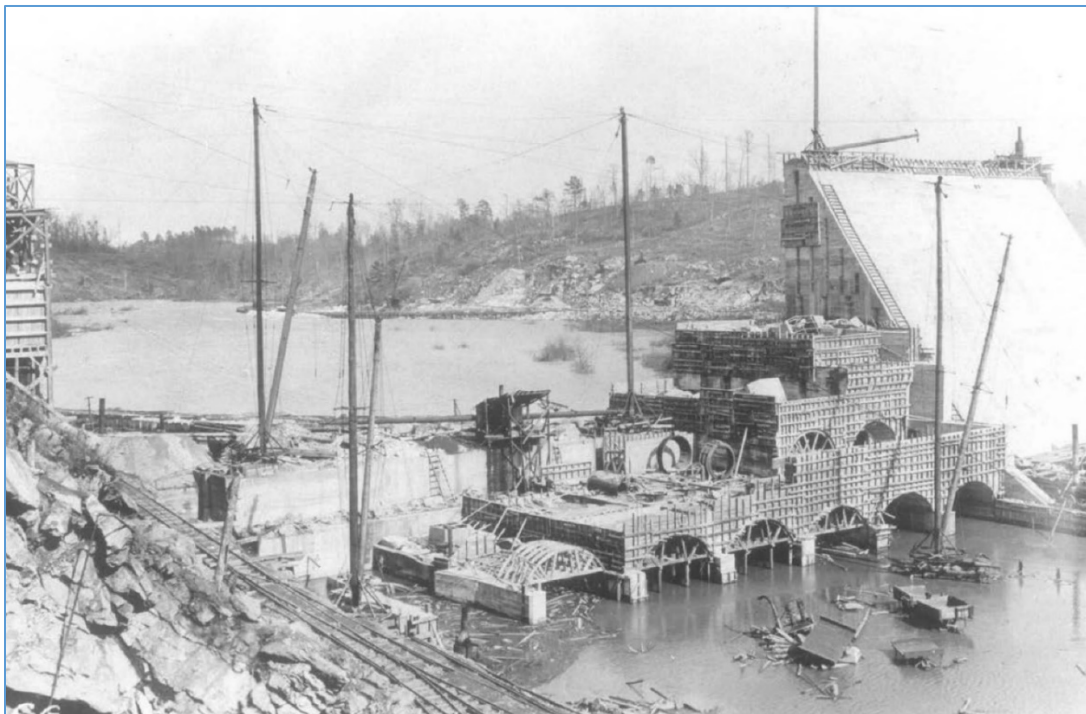
Figure 3. Lloyd Shoals dam and powerhouse under construction circa 1909, looking northeast (Courtesy of Georgia Power).
