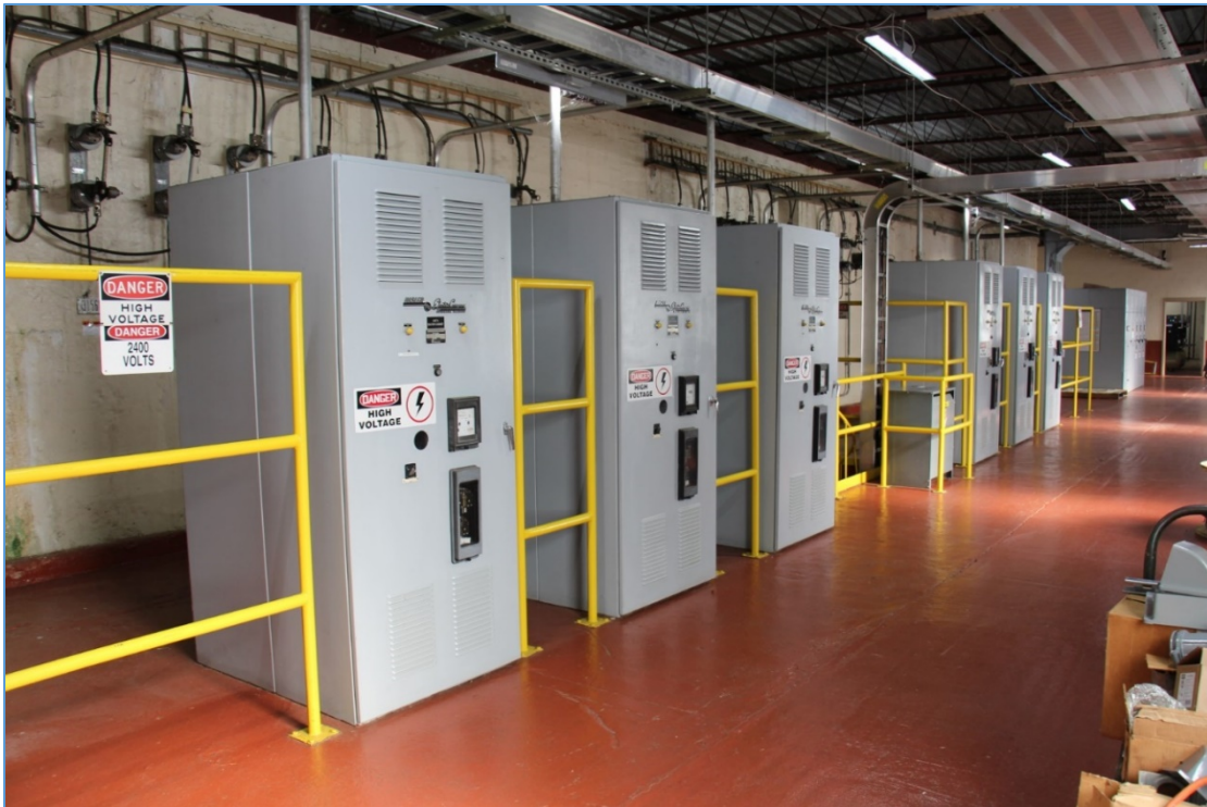
Figure 19. Interior view of second floor showing electrical equipment, looking northeast, December 2, 2019.
